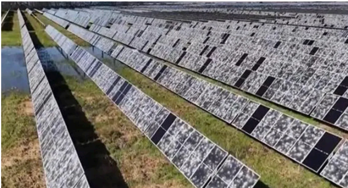
Solar panels in Fort Bend County, Texas, were heavily damaged last month during a hail storm. Photo: Fox 26
